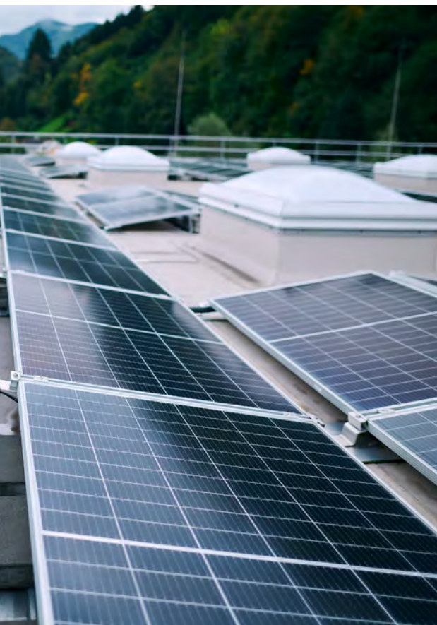
← Photovoltaics system at the Marktl site
